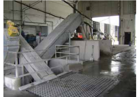
PDC Pump Discharge Conveyor charging BIBKO® 1000
