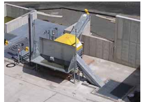
Concrete Pump Washout "PDC" module
